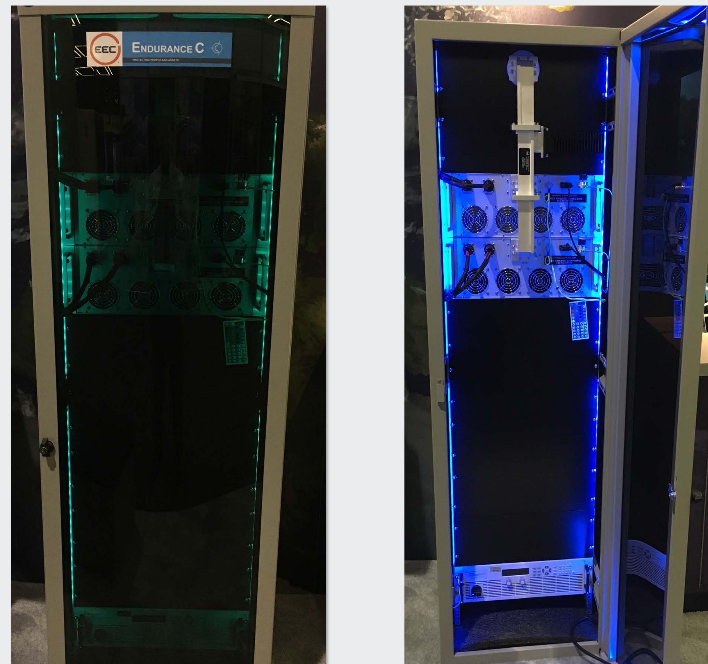
Endurance C Transmitter Cabinet (shown here with only two of the final four operational 2.5 kW amplifiers bays)
